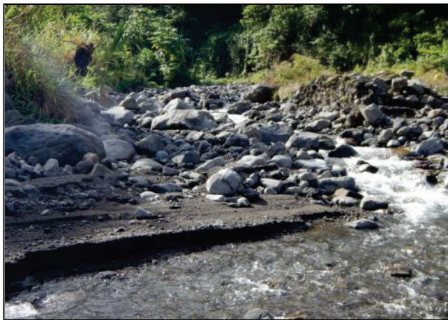
Figure 4-15: Rabacca River Upstream of Damaged Intake during Site Visit on February 2016
